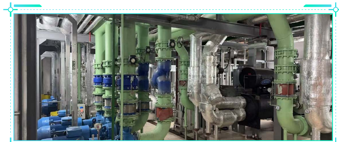
The headquarters building adopted a lower energy-consuming water storage central air conditioning cooling system
